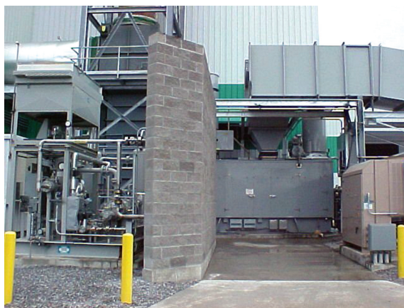
Turbine generator for gypsum wallboard manufacturer.
