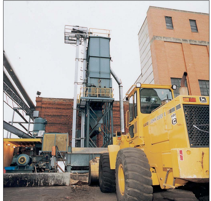
50-ton/hr chipper, 10-ton storage silo and conveyer system are used to convert waste wood to solid fuel for co-firing with coal.
