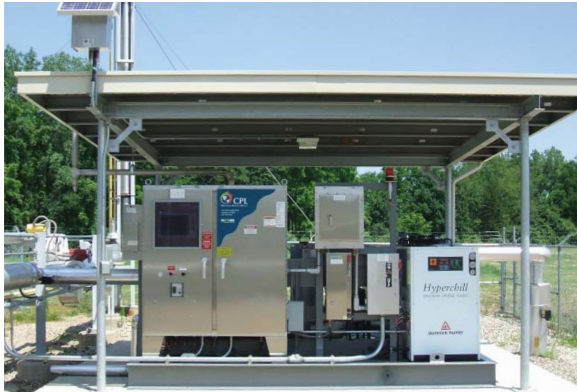
CPL Biogas Skid
