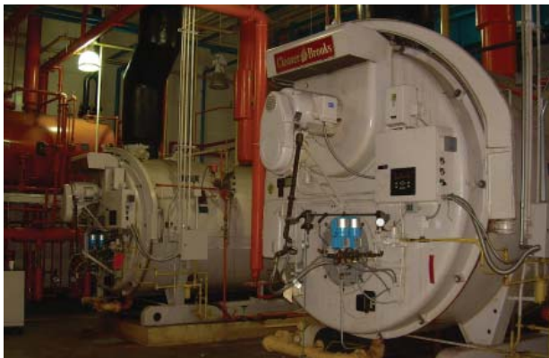
Typical Boiler Room
