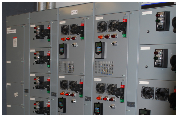
Main Control Room
