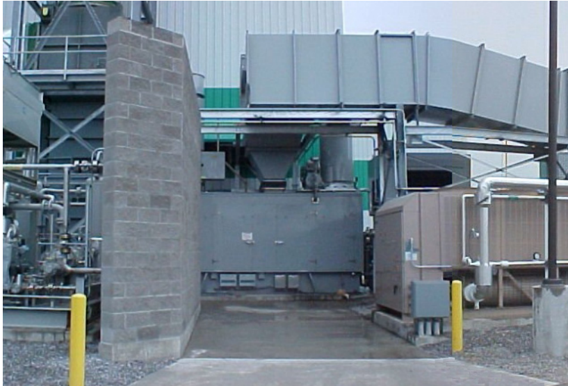
Turbine Generator Set
