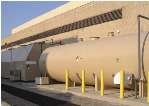
Fuel Oil Storage Tank
