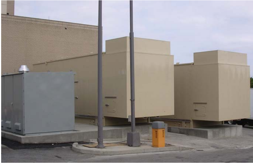
Switchgear and Generators
