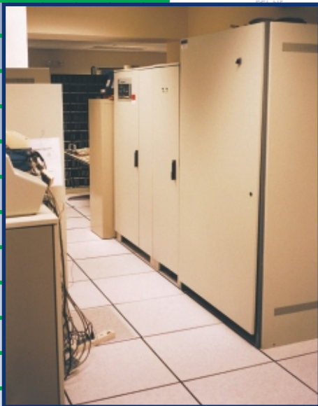
Data Center Power System
