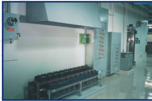
125-Volt DC Battery, Charger and Switchboard
