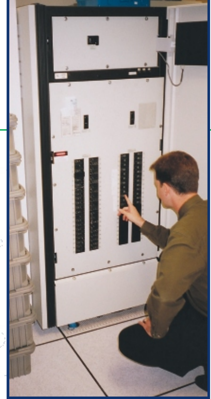
Computer System - Power Distribution Unit
